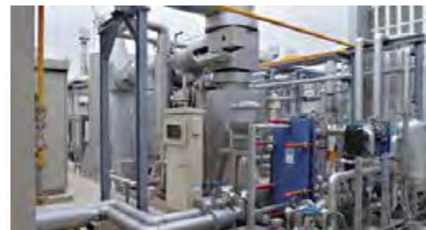
An environment-friendly cogeneration system using natural gas at our Gunma Factory
